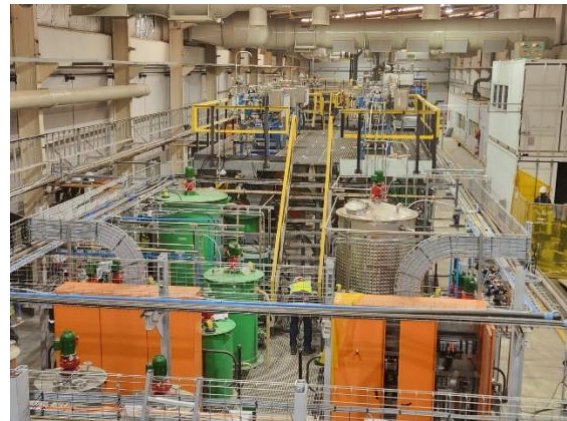
Figure 3. Overview of the Demo Plant
