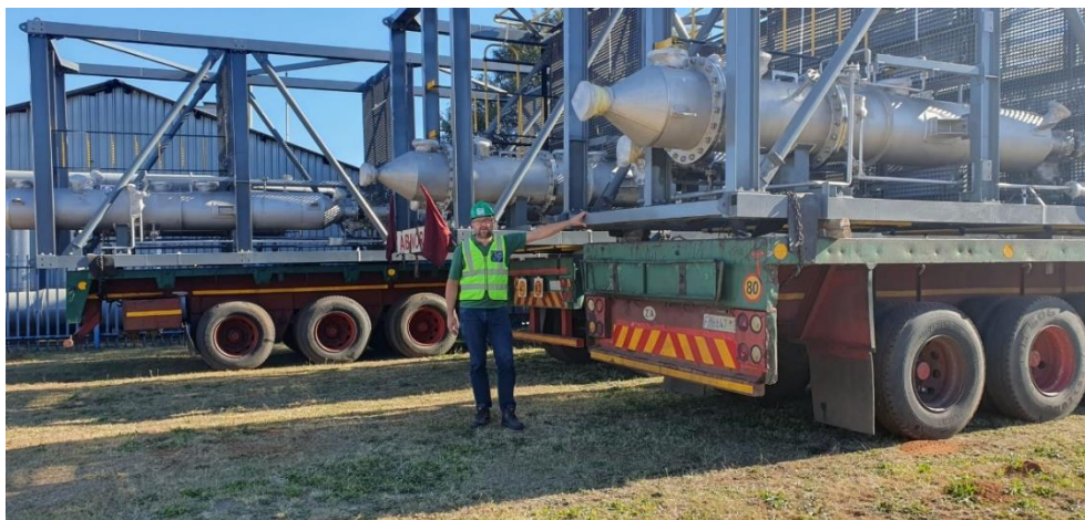
Figure 1 VP, Project Development & Construction Dirk Geerligs overseeing the delivery of the Crystallizer Unit to the Demo Plant Site in Johannesburg
