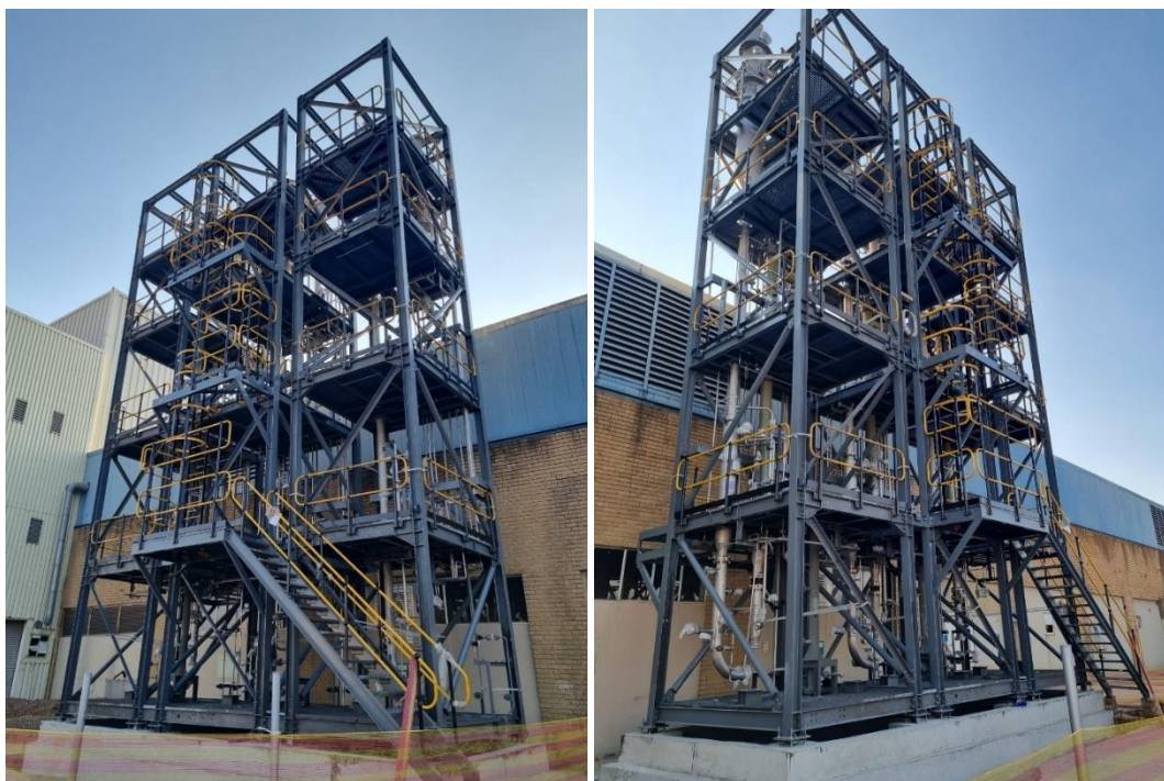
Figure 2 Crystallizer unit installed at Demo Plant site in Johannesburg, South Africa
