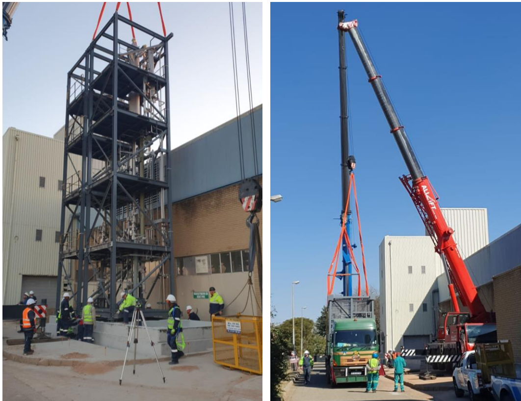
Figure 4 Installation of the crystallizer unit, which is comprised of two crystallizers and an evaporator.
