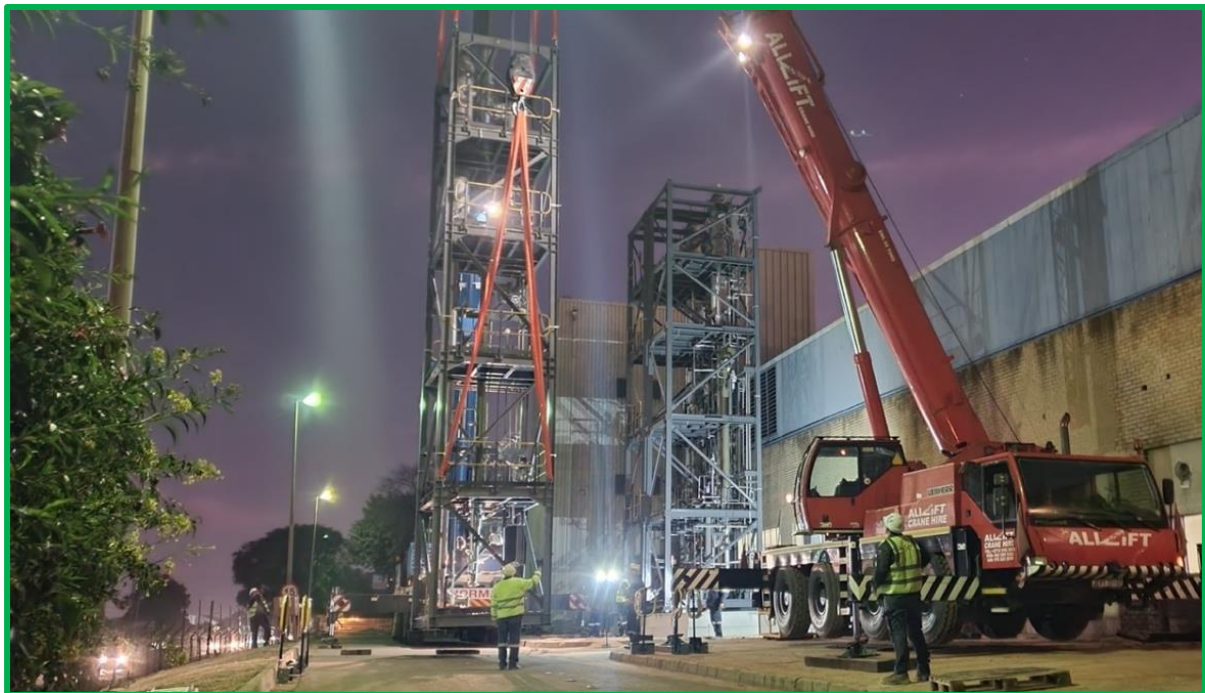
Figure 2: Crystallizer Installation in 2023
